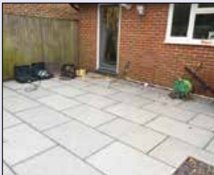
Ensure you have prepared a level concrete base or a properly fitted existing patio or decking.
